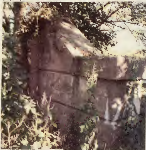
Fig. 55 Close-up view of surviving trestle in the village of Pikeland. •Local sources said that Mr. Hallman, the owner of the local store and the property on which the trestles sit, was offered a suitable sum of money by the railroad company so they would not have to go to the trouble of having the piers removed. Photograph by the author, 1995.
